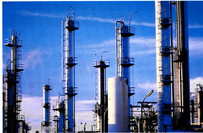
Crude oil is separated into fractions by distillation in cylindrical towers typically 8 m in diameter and 40 m high
